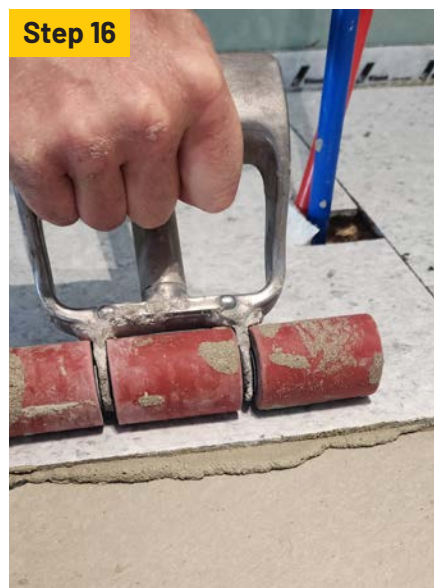
Use hand or large embedding rollers or flat trowels to achieve 100 % mortar transfer.
